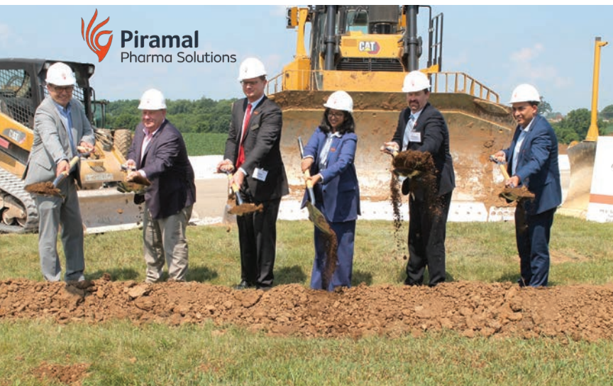
In June 2025, Piramal Pharma Solutions broke ground on the expansion of its Lexington facility, which specializes in sterile compounding, liquid filling, and lyophilization for sterile injectable drug products. (Photo by Commerce Lexington staff)
